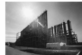
Figure 5. Savannah River heavy water plant's 130 foot tall distillation towers.
