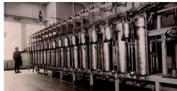
Figure 4. Norsk Hydro 18 electrolysis cells at Vemork. Source: Nova.
