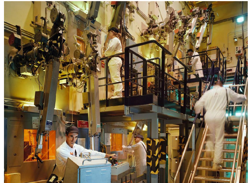
AREVA reprocessing plant, France (courtesy of AREVA)
