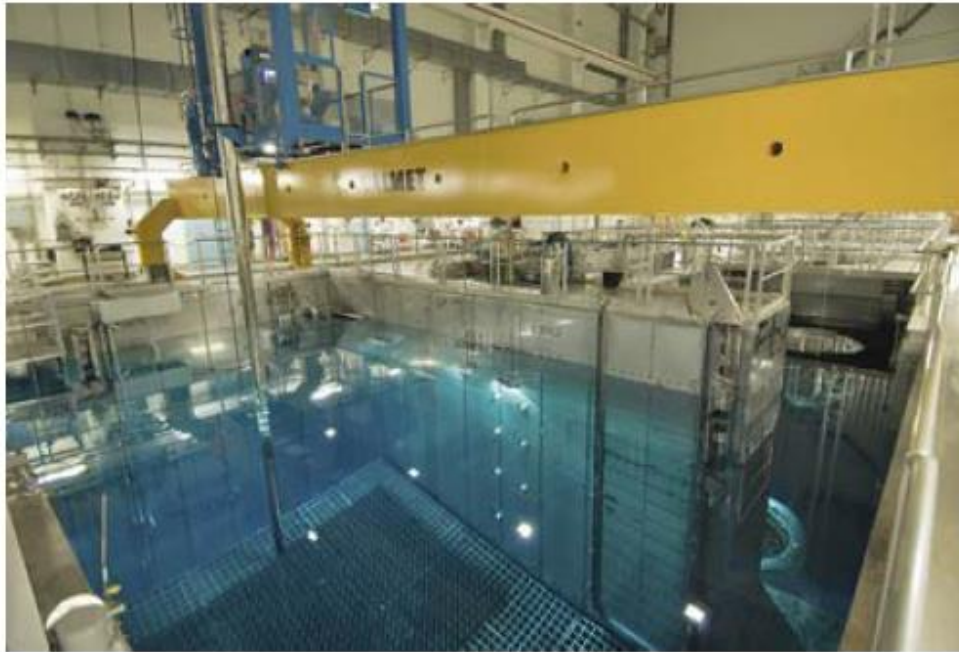
Wet storage facility at the Olkiluoto NPP (Finland)
