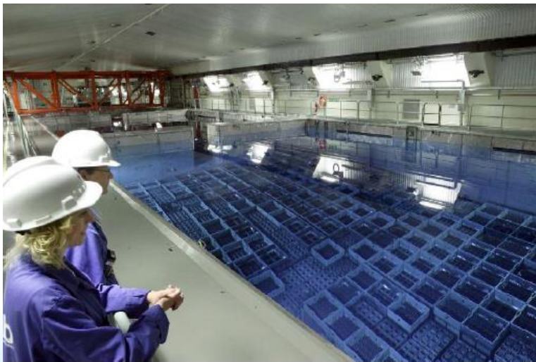
The interim storage of spent fuel at Clab, Sweden (courtesy of SKB)
